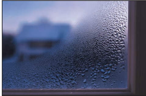
Condensation on the inside of a windowpane.
