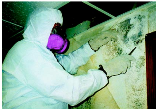
Photo 7: Remediation worker with limited PPE
