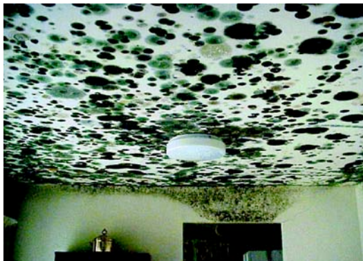
Photo 2: Extensive mold contamination of ceiling and walls
