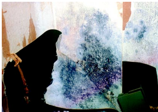
Photo 5: Mold growth behind wallpaper
